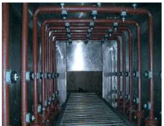
SPRAY HEADERS & SYSTEMS
